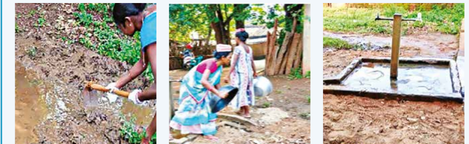
A group of determined women sanitation leaders engage in shramdaan, working to maintain hygiene and cleanliness around a drinking water standpost in their community
