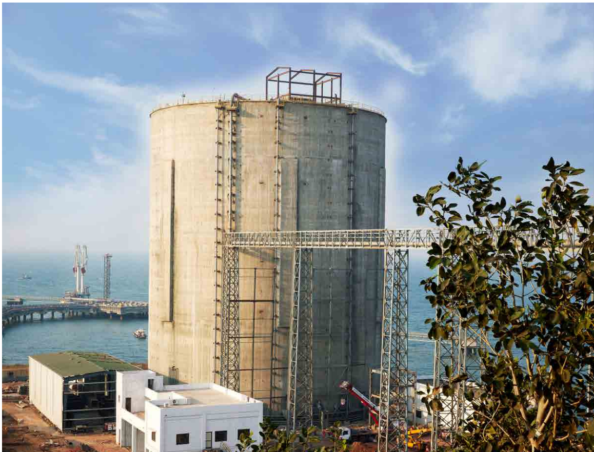
Completed the construction of 45,000 MT Ash Silo of JSW Energy at Ratnagiri JSW Port
