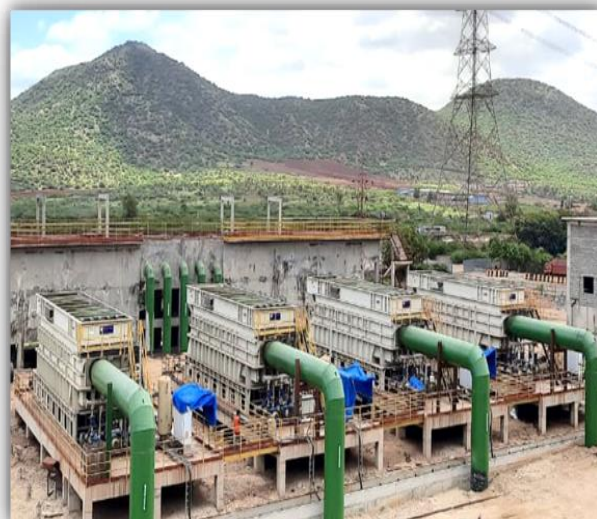
Raw water Treatment Plant-2
