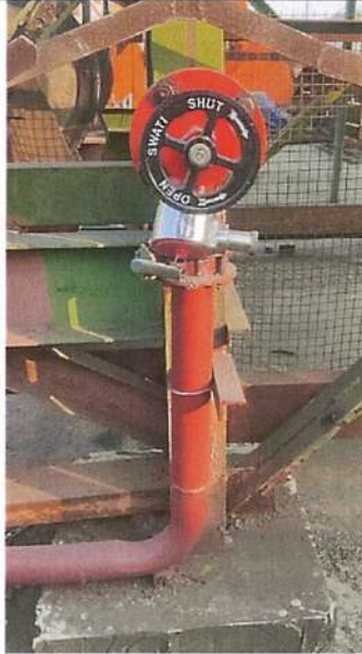
Fire hydrant post
