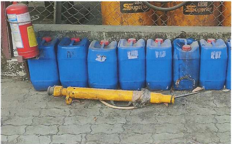
200 liters of Foam making compound, sand buckets & extinguishers
