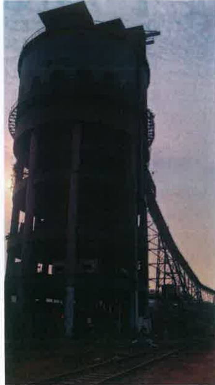
Silo loading attached with pipe conveyor
