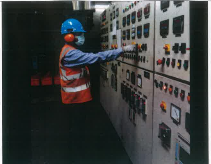
Ear muffs provided for Person working near DG.
