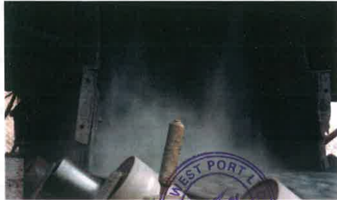
Mist System in hoppers
